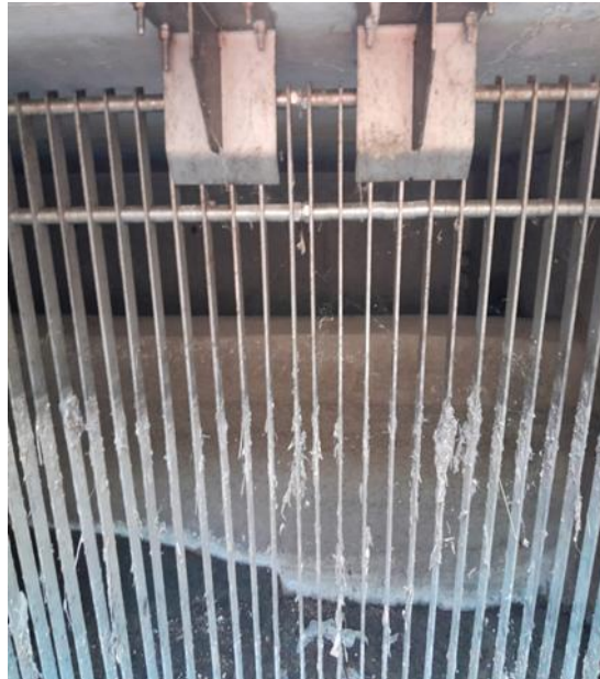
SWO1-Storm Water Overflow
