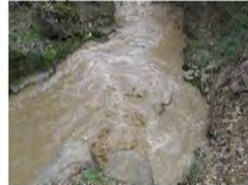
New discharge point 17
